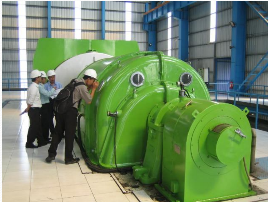
Generator dan Steam Turbine
