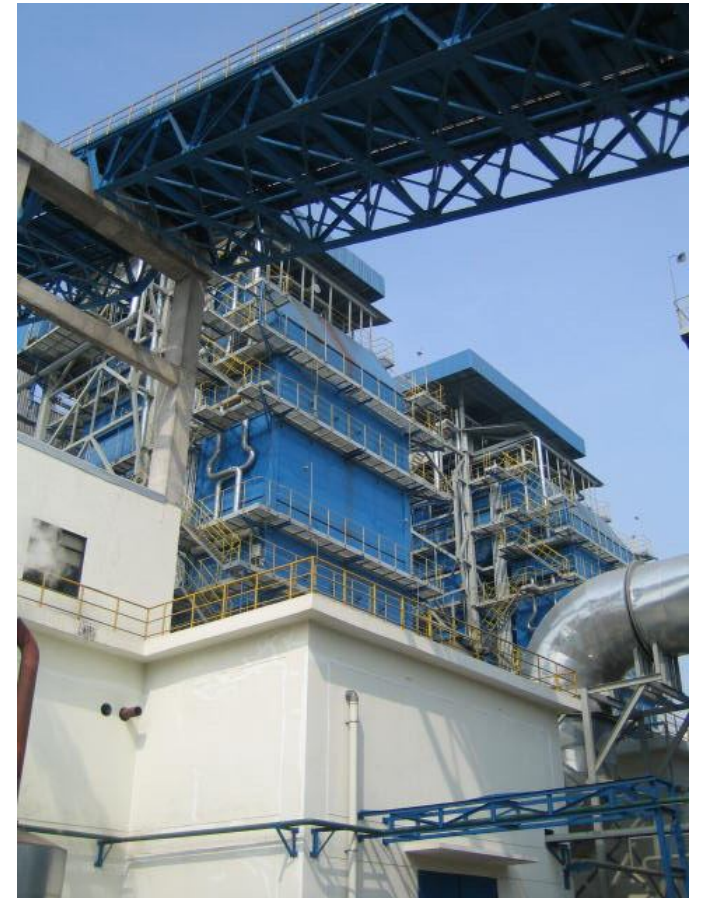
Fluidized Bed Boiler
