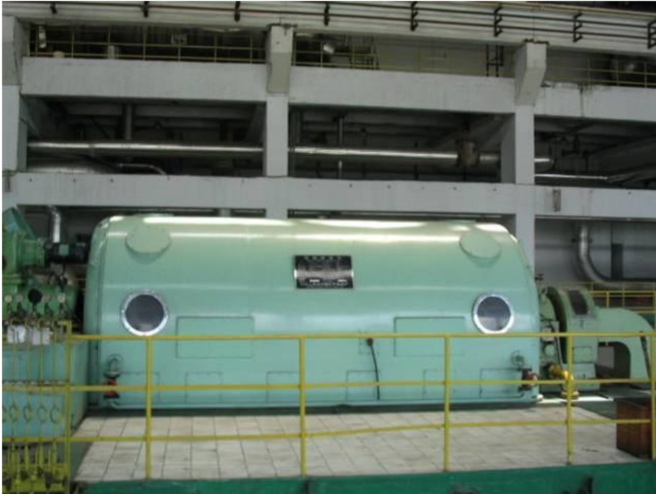
Steam Turbine Generator
